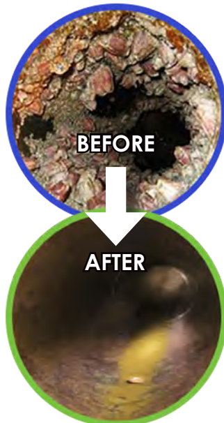
Water Piping Scale
