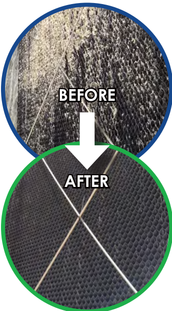
Cooling Tower Scale
