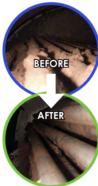
Heat Exchanger Scale
