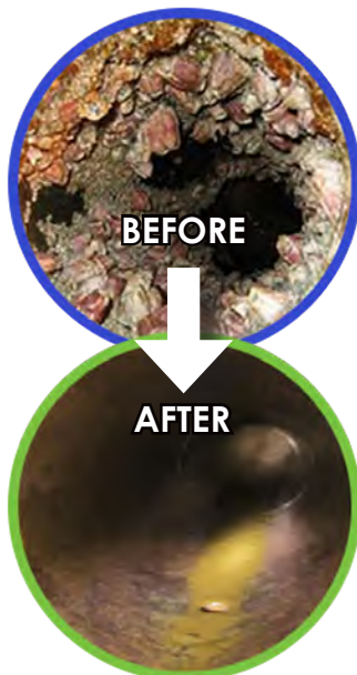
Water Piping Scale
